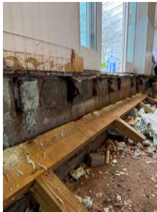
Sill on waterside collapsing, temporary support to hold it up, all joists rotted
